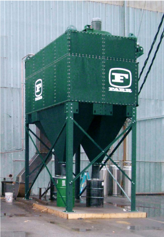
Farr Gold Series GS24 installed at Chatham Steel on a plasma cutting table application.
