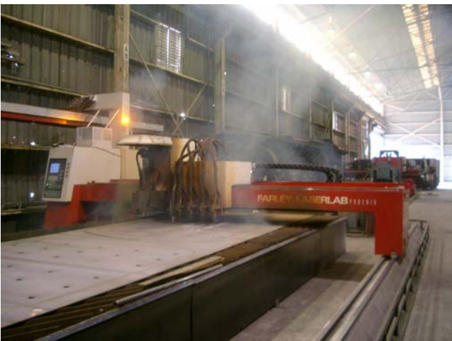
Before Farr Gold Series collector was installed - smoke from plasma cutting operation filled the facility.
