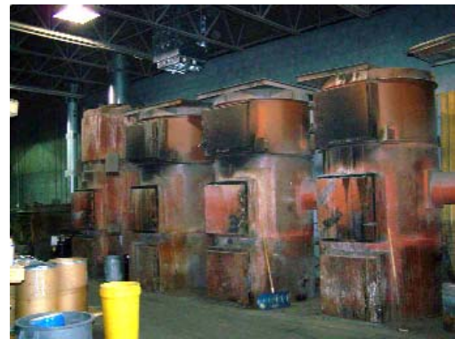
Fumes from incinerators are captured by the Gold Series after being cooled through the duct work with outside air.
