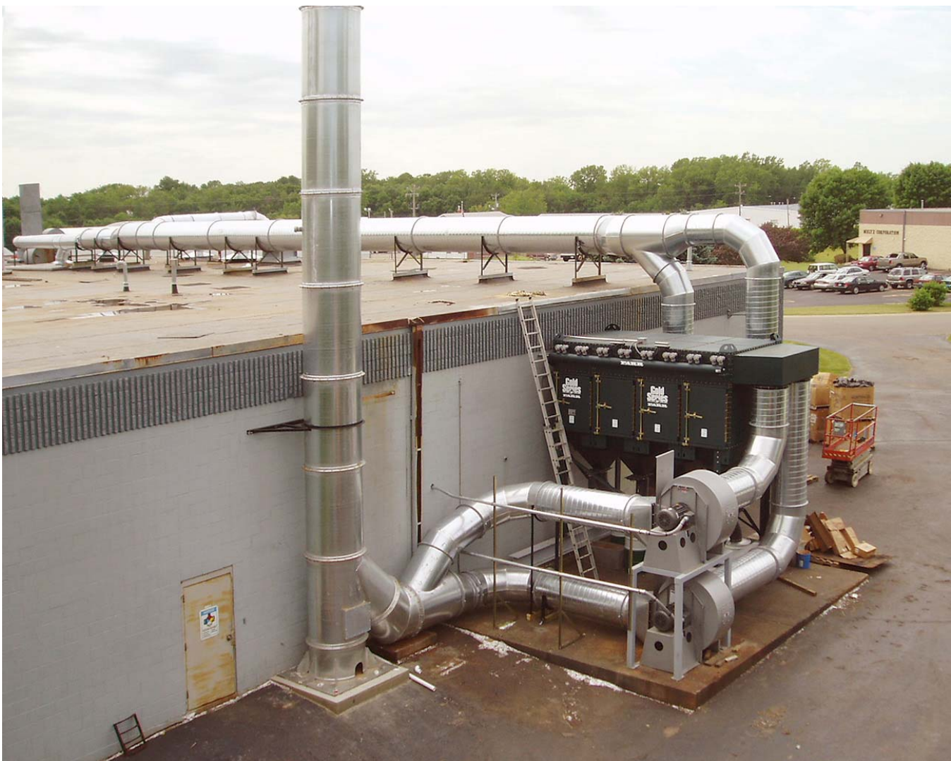
32,000 CFM through the Gold Series provided by twin fans controlled by a variable frequency drive (VFD).
