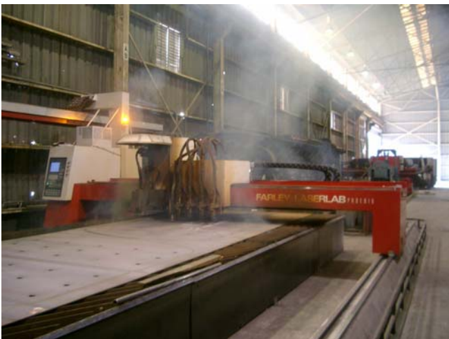
Before Farr Gold Series collector was installed - smoke from plasma cutting operation filled the facility.
